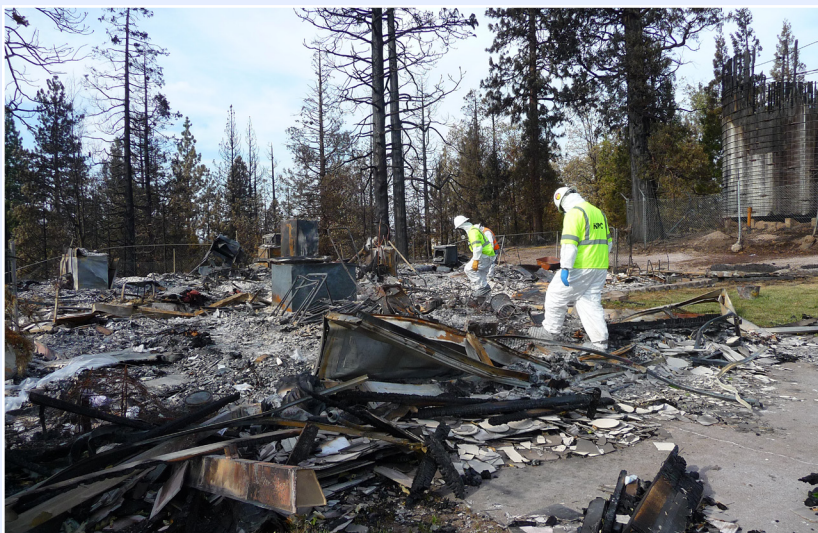
Left: Contractors search for hazardous material among the ruins of a building.
