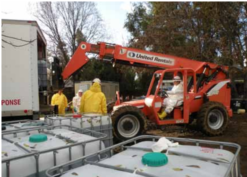
Workers prepare to haul dangerous chemicals from an orphan site in Yuba County.
