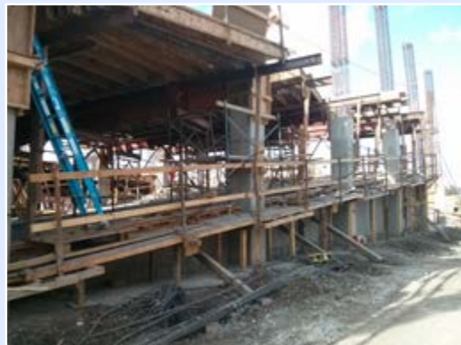
Above: an office building and parking garage rise as part of the Santa Clara Square project.
